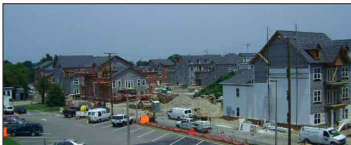
Construction of innovative military housing is underway on three sites in Hampton Roads.
